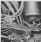
Junction Block Shut-off Valve and Accumulator Tank Shut-off Valve—(Turn clockwise to close; counter-clockwise to open)
